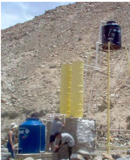
Fig. 3. Huayash solar-pumped water system sand filters.
